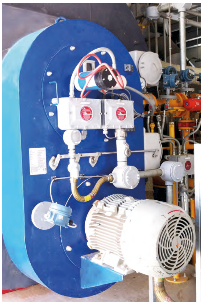
Burner adapted to the ATEX explosion proof regulations. Source: E&M Combustion
